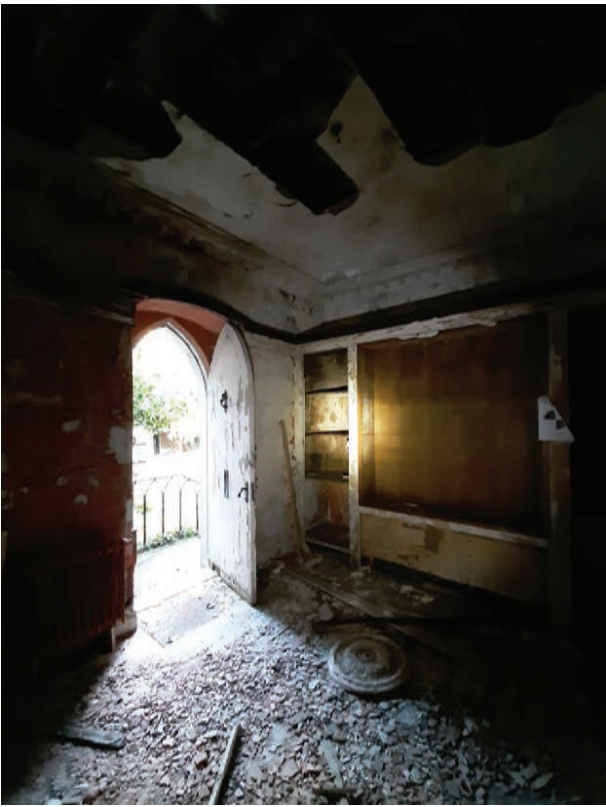
Ground floor of the tower with existing timber entrance door still in place. Note this door will be retained and refurbished.
