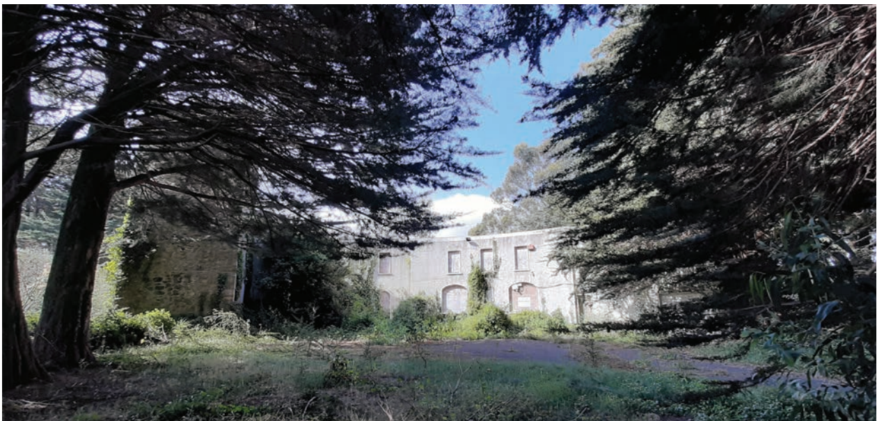
View of the current condition of the house and tower from the north
