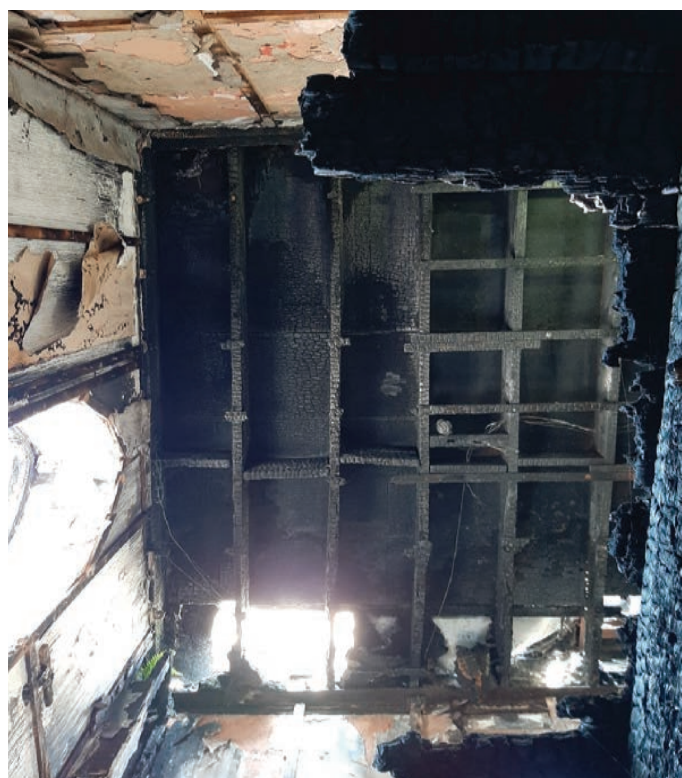
Fire damaged timber floors and stairs to be removed from the tower
