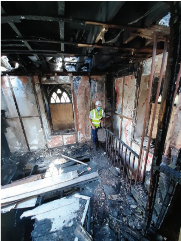
Second floor of the tower - charred timbers throughout
