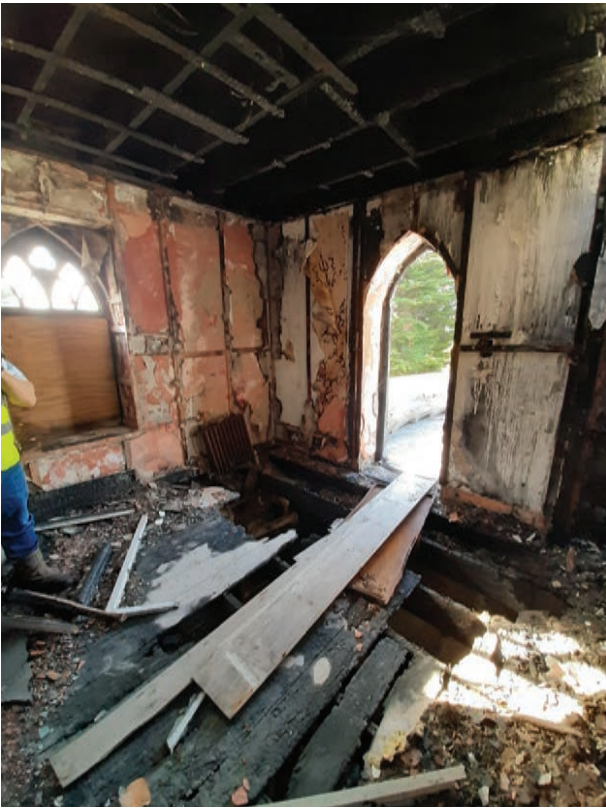
Second floor of the tower looking towards the flat roof of the house
