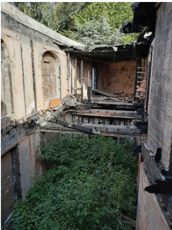
Poor condition of the house
