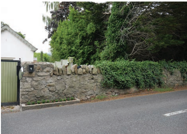
Existing stone wall on southern side of Brennanstown Road where it meets the adjoining residential property to the east of the site.
