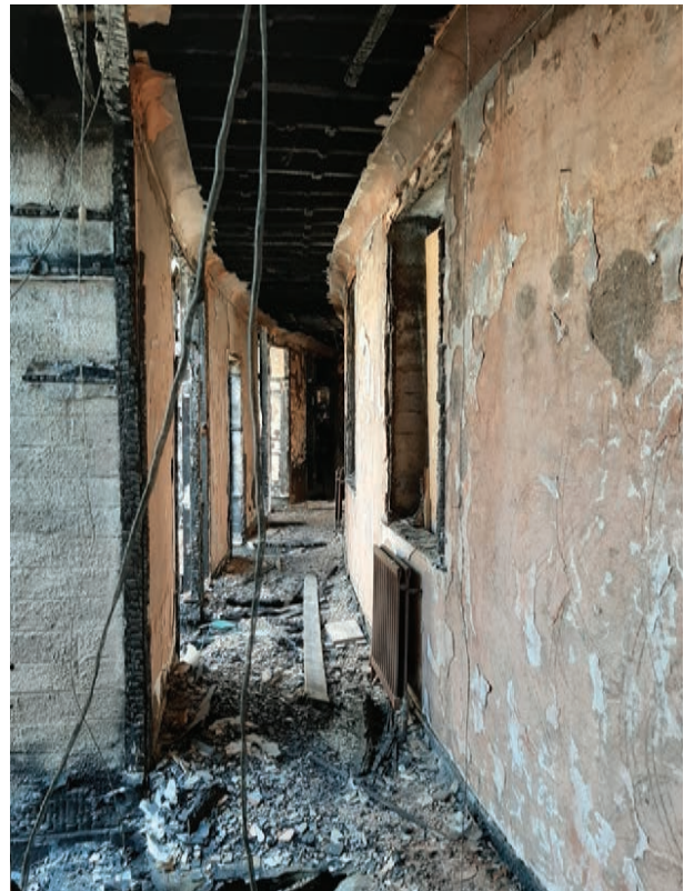
Poor condition of internal corridor
