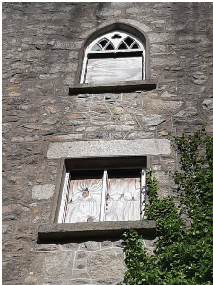
Window surrounds and lintels to be retained and repaired with new timber windows designed to match profile of existing windows on site
