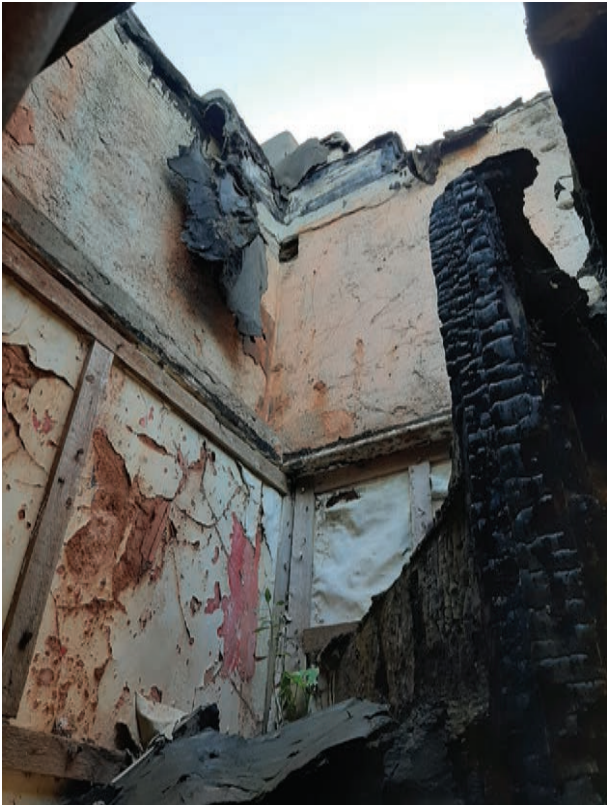
Parapet roof of the tower with failing asphalt, and top of charred timber staircase shown on the right
